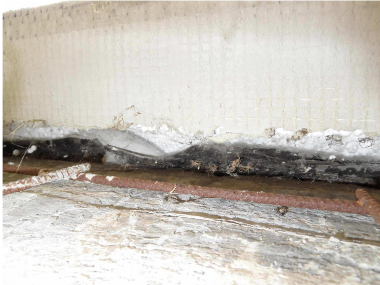
Figure 1: Gap between peripheral wall and its heat insulation, incorrect gluing of heat insulation boards
