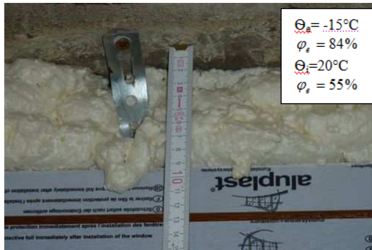
Figure 4: Gap size between the window and the reveal 10 cm.
