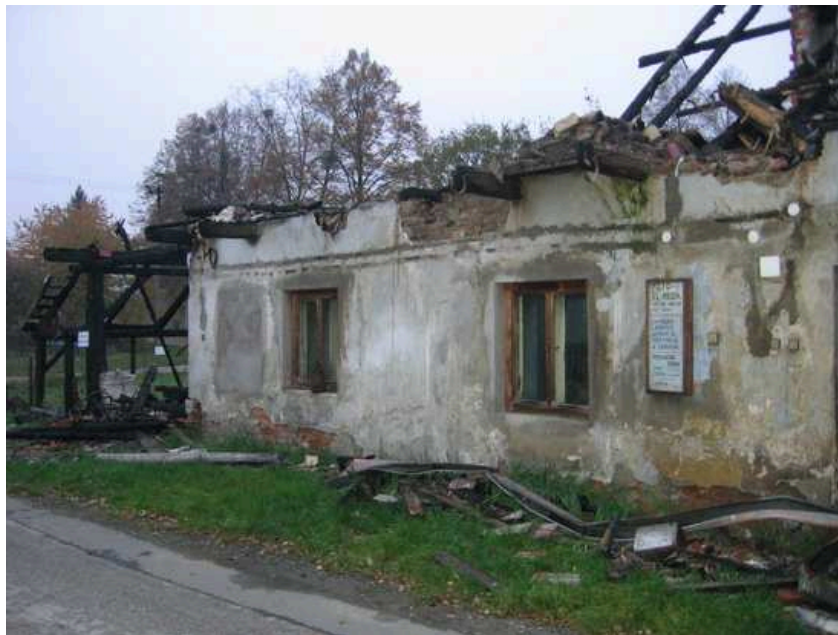
Fig. 1: The building damaged by fire
