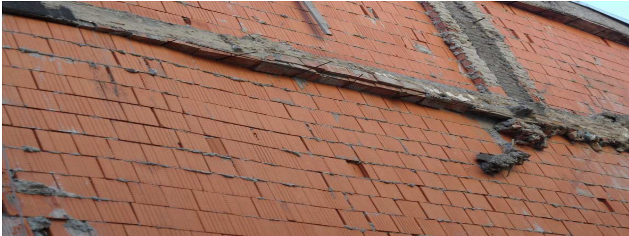
Figure 1: Damaged bearing structure of the building, which are assessed in tab. 2
