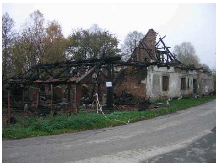
Fig 1 : Building damaged by arson
